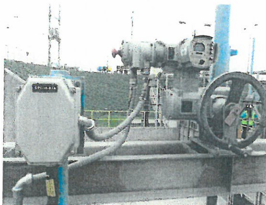
COMPUERTAS MOTORIZADAS (BYPASS) CM-10-01 A
